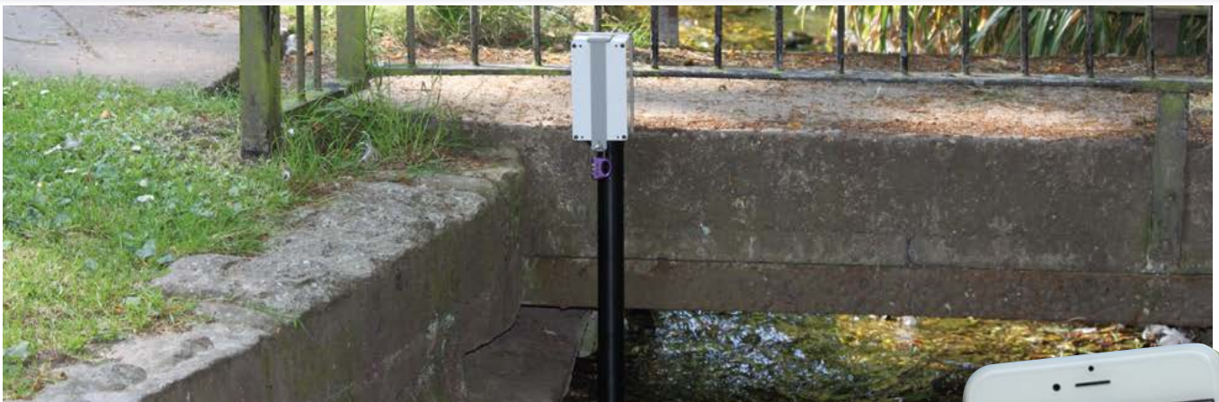
LevelLine-EWS deployed along a shallow riverside
